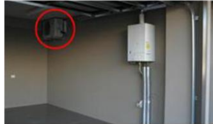
Air conditioning plant located within garage
