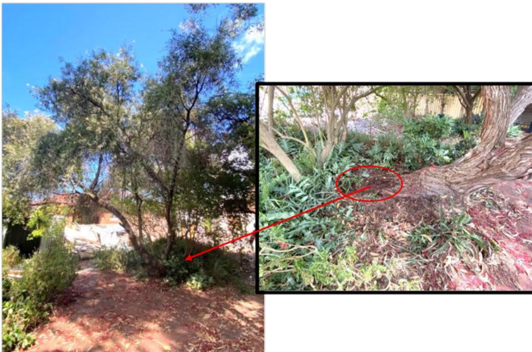
Figures 3 & 4 Displaying Tree 1, a Callistemon viminalis within the rear yard of 23 Monk St, Kensington and indicating evidence of minor root heave.
