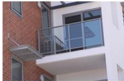
Screened balcony mounted air conditioning plant located at floor level.
