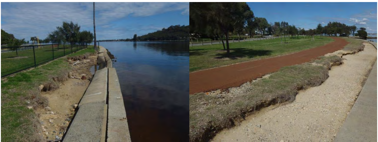
Plate 4: Erosion damage along Narrows foreshore a) to river walling and b) threatening footpath
