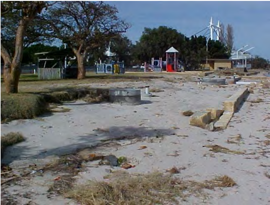
Plate 2: Damage at Como Beach after May 2003 storm.
