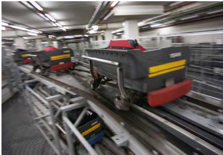
Luggage moves on rapid-speed conveyors
