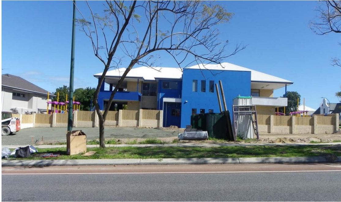
The site as viewed from Labouchere Road with the approved Child Day Care Centre under construction
