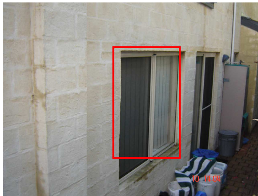
Figure 2 - photograph of the habitable room window (marked in red) on the adjoining property.
