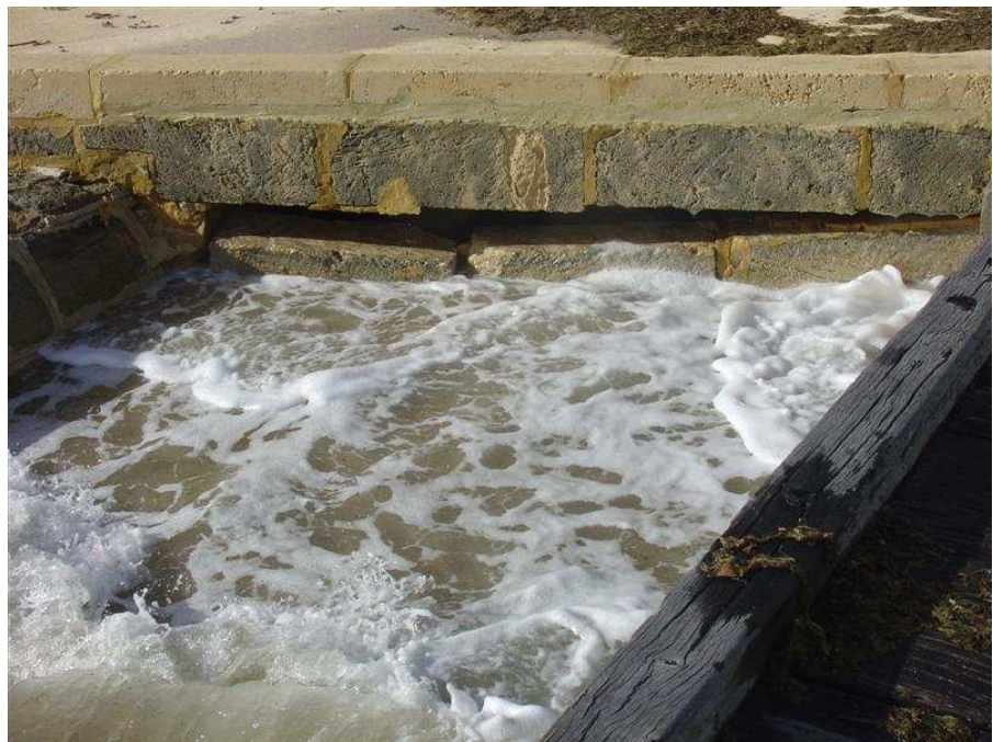
Figure 2. Wall damage adjacent to jetty, Como Beach - July 2008
