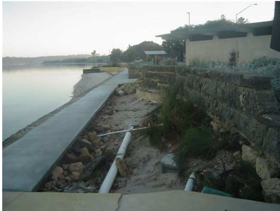
Figure 3. Result of wall damage, Como Beach - July 2008
