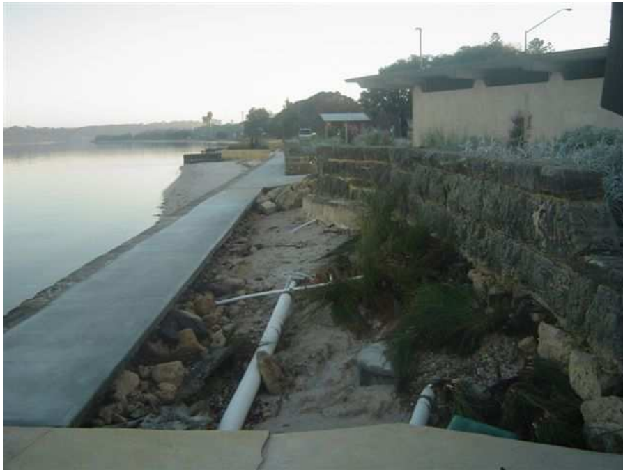
Figure 3. Result of wall damage, Como Beach - July 2008
