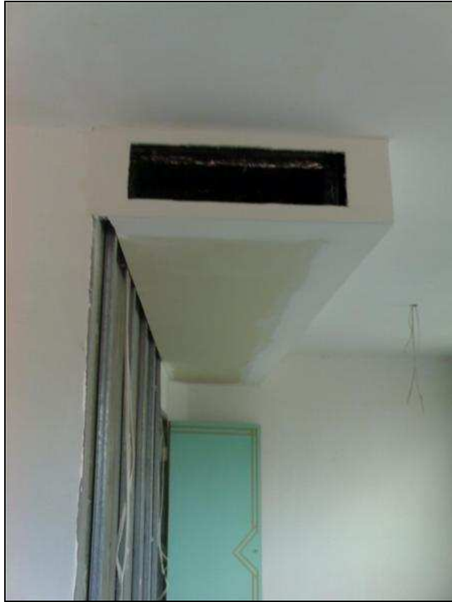
Figure 7: Air-conditioning spur duct and vent to Level 4 “Balcony”.
