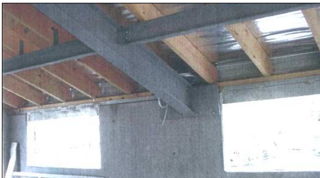
Figure 5: Unauthorised over-height modification (internal) to concrete wall panel.
