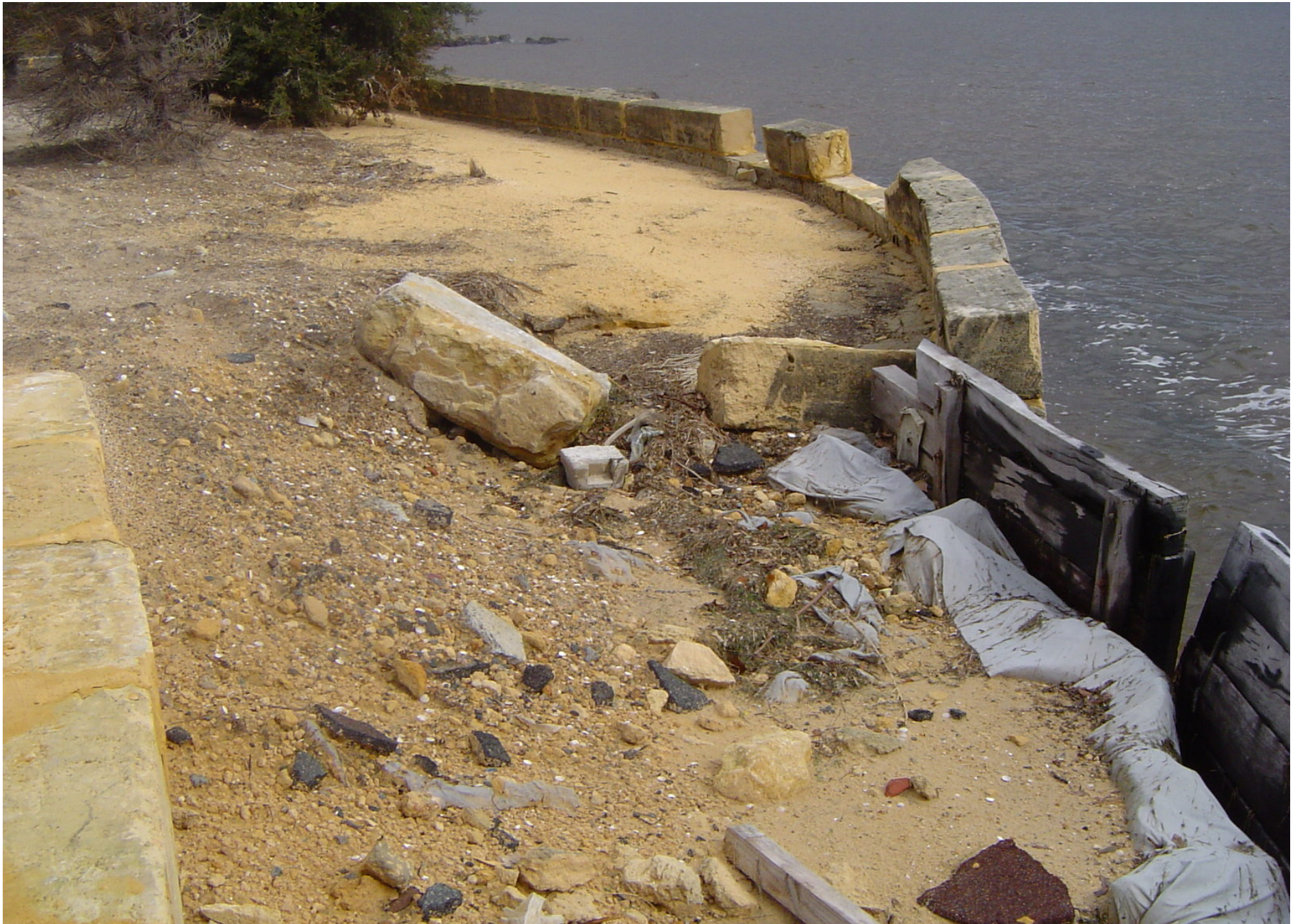
View of failing wood wall section
