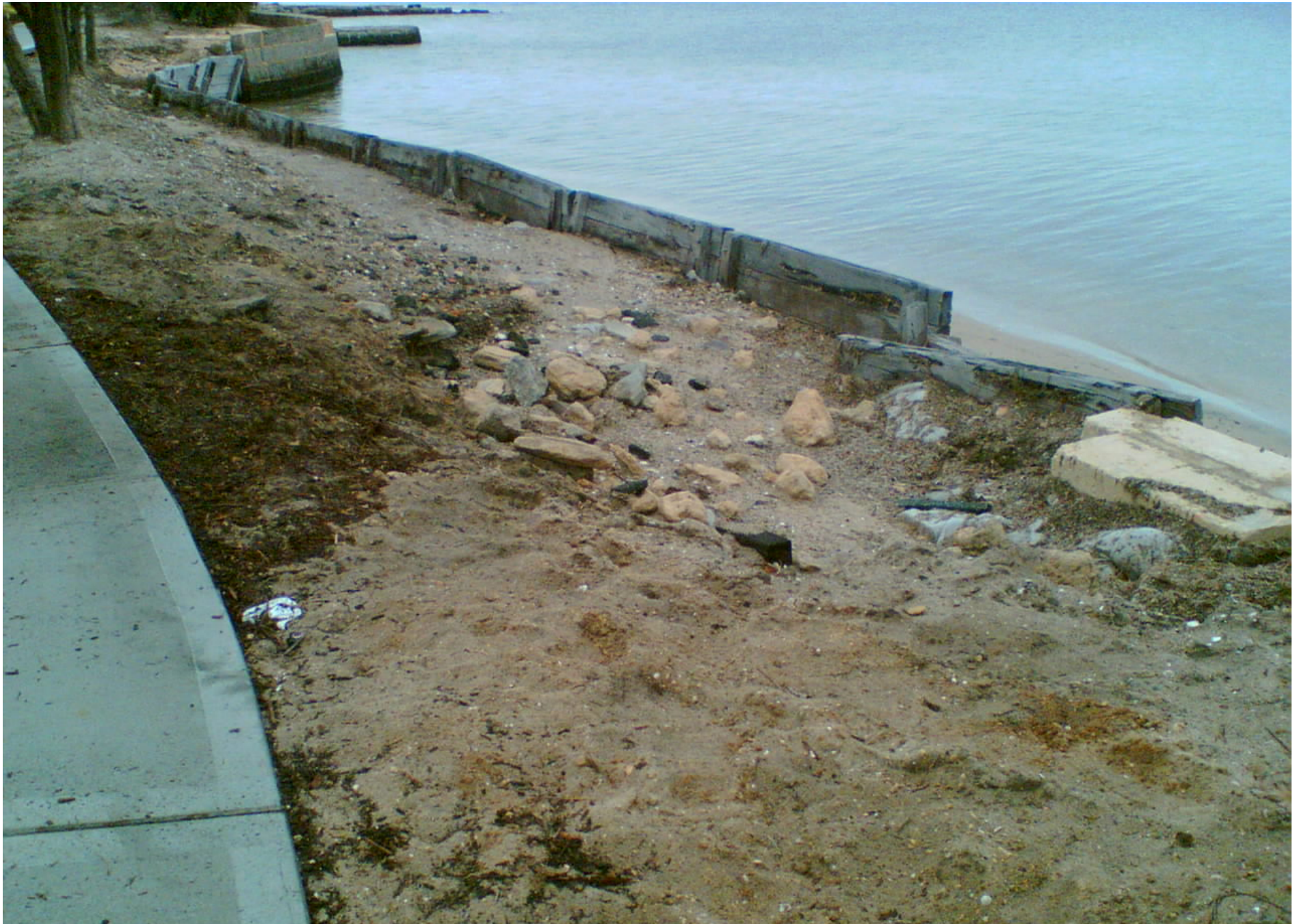
View of failing wood wall section
