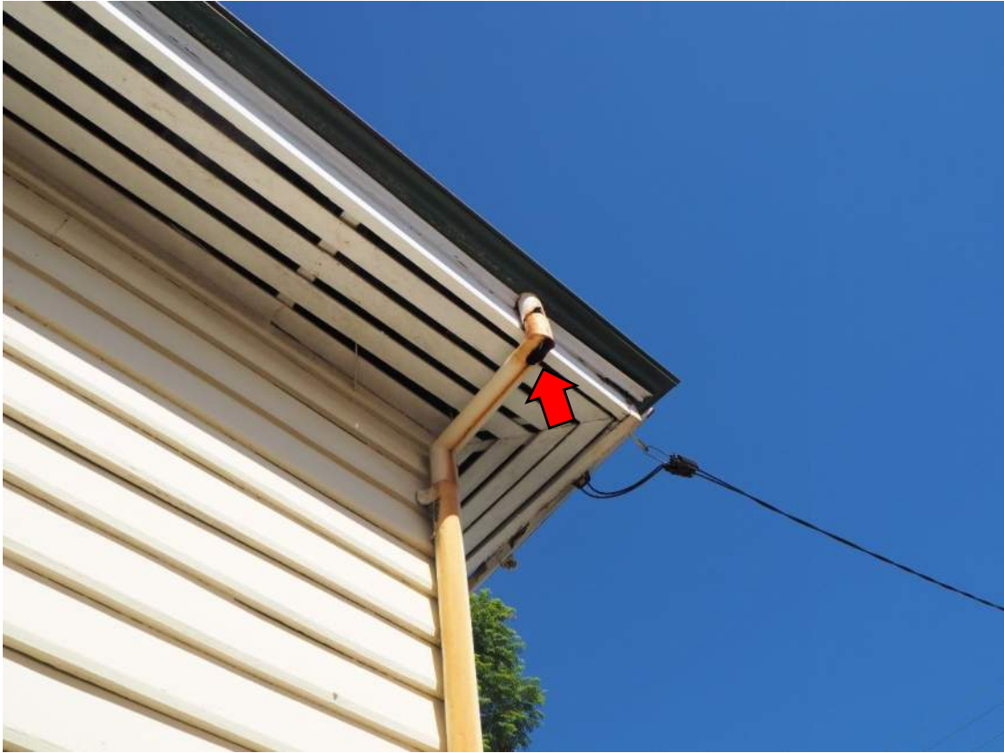
Photo 23 – Severely corroded downpipe.
