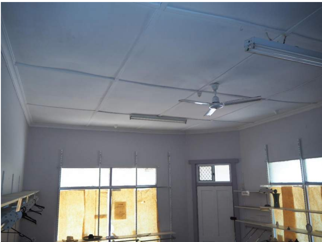
Photo 26 - Ceiling sagging in corner shop
