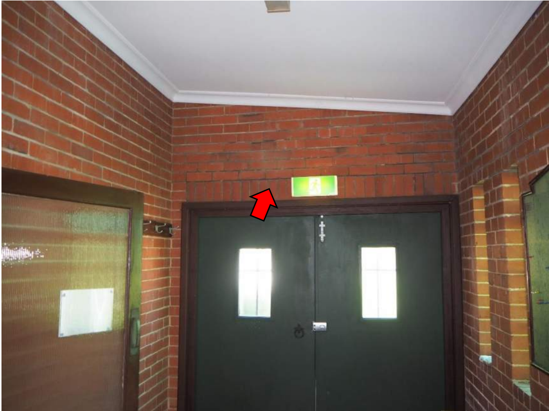
Photo 13 – Different coloured pointing above doorway.
