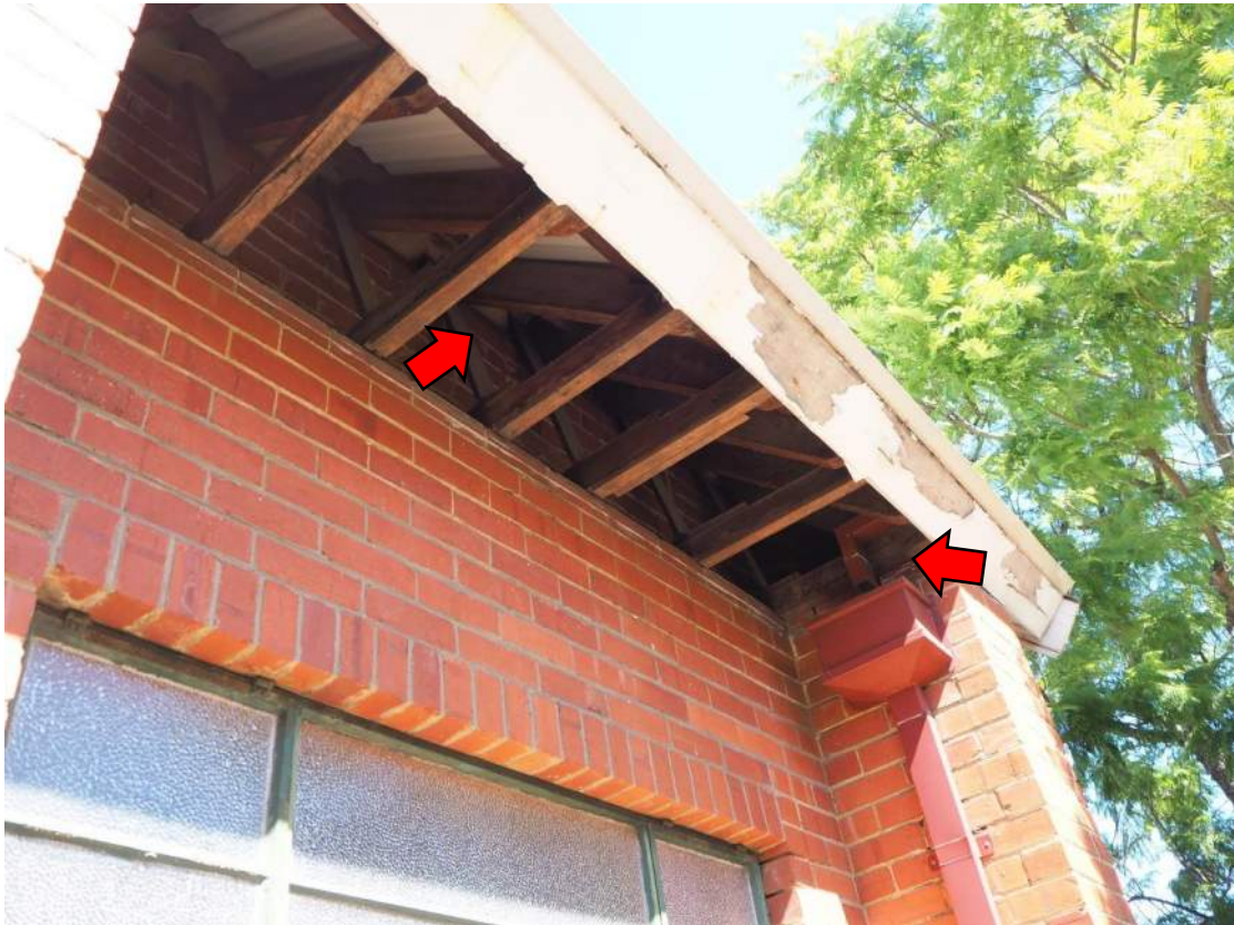
Photo 07 - Missing eaves boards. Note connection between hidden eaves gutter and downpipe rain head.
