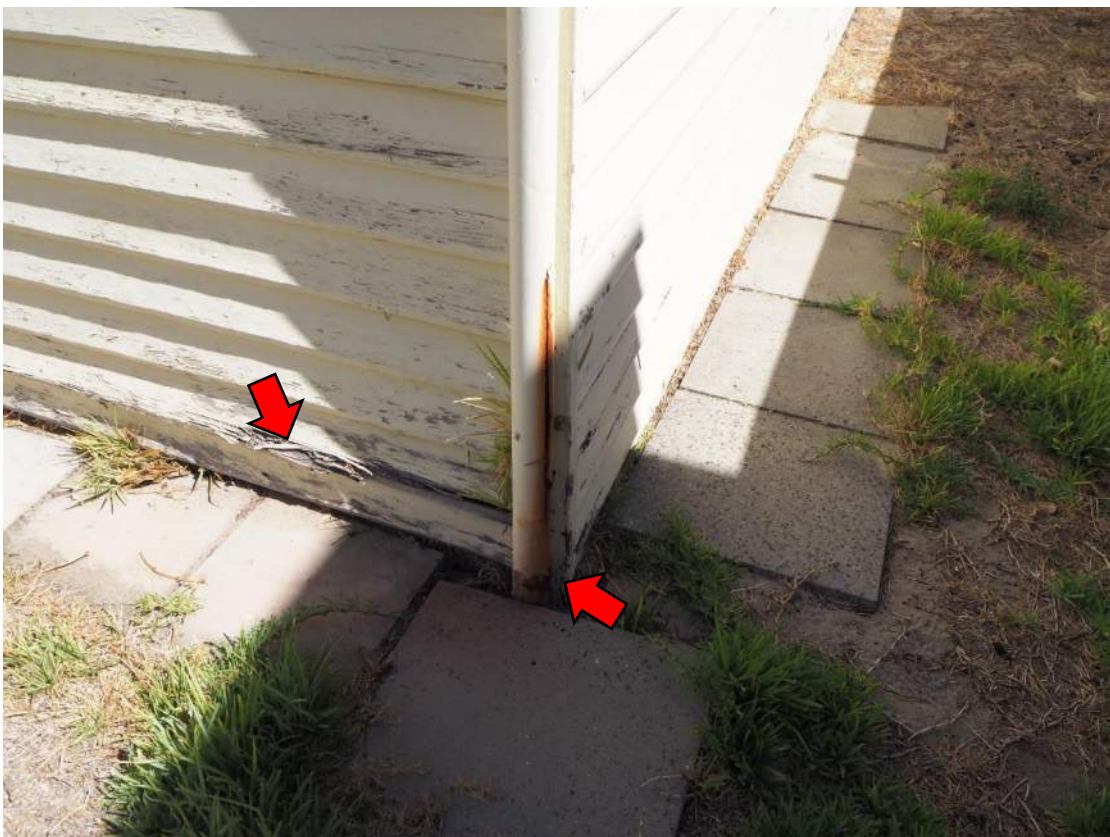
Photo 22 – The timber weatherboard was badly weathered in places and the downpipe was corroding and discharging directly onto the ground.
