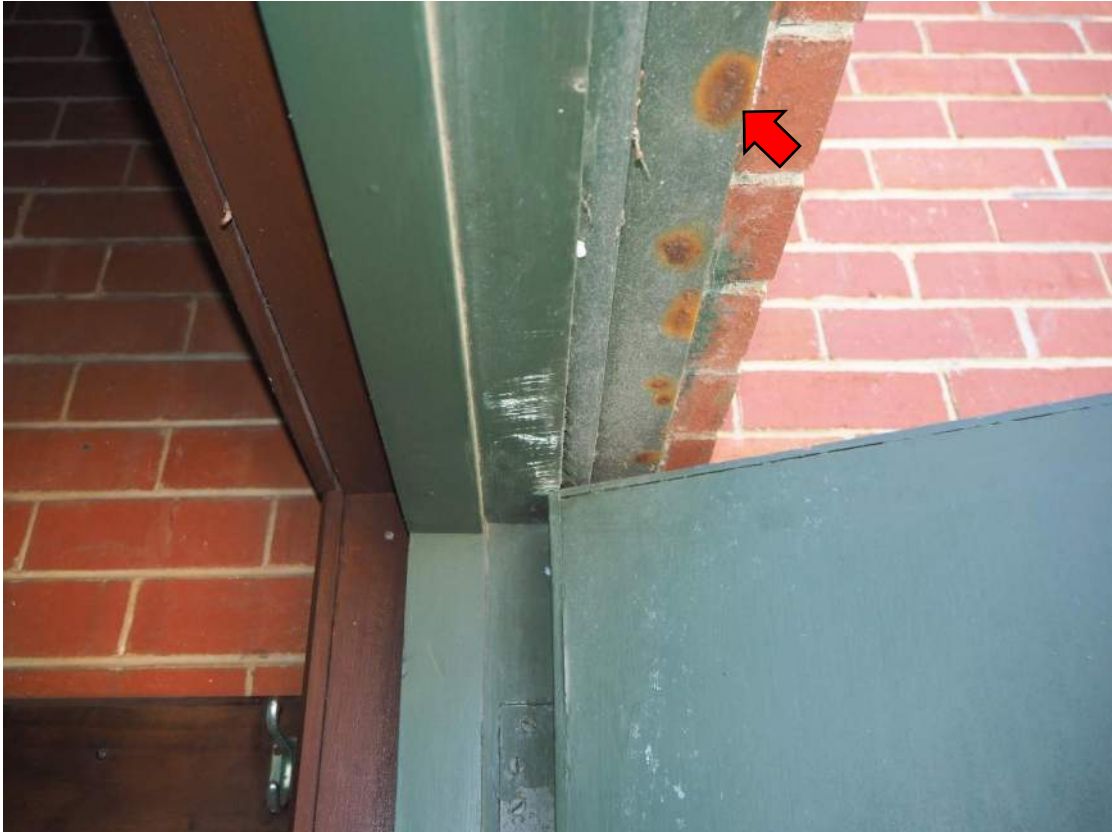
Photo 15 – Corroding lintel over doorway
