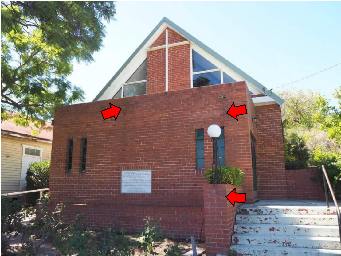
Photo 02 – Fretting mortar and damp staining, southwest elevation
