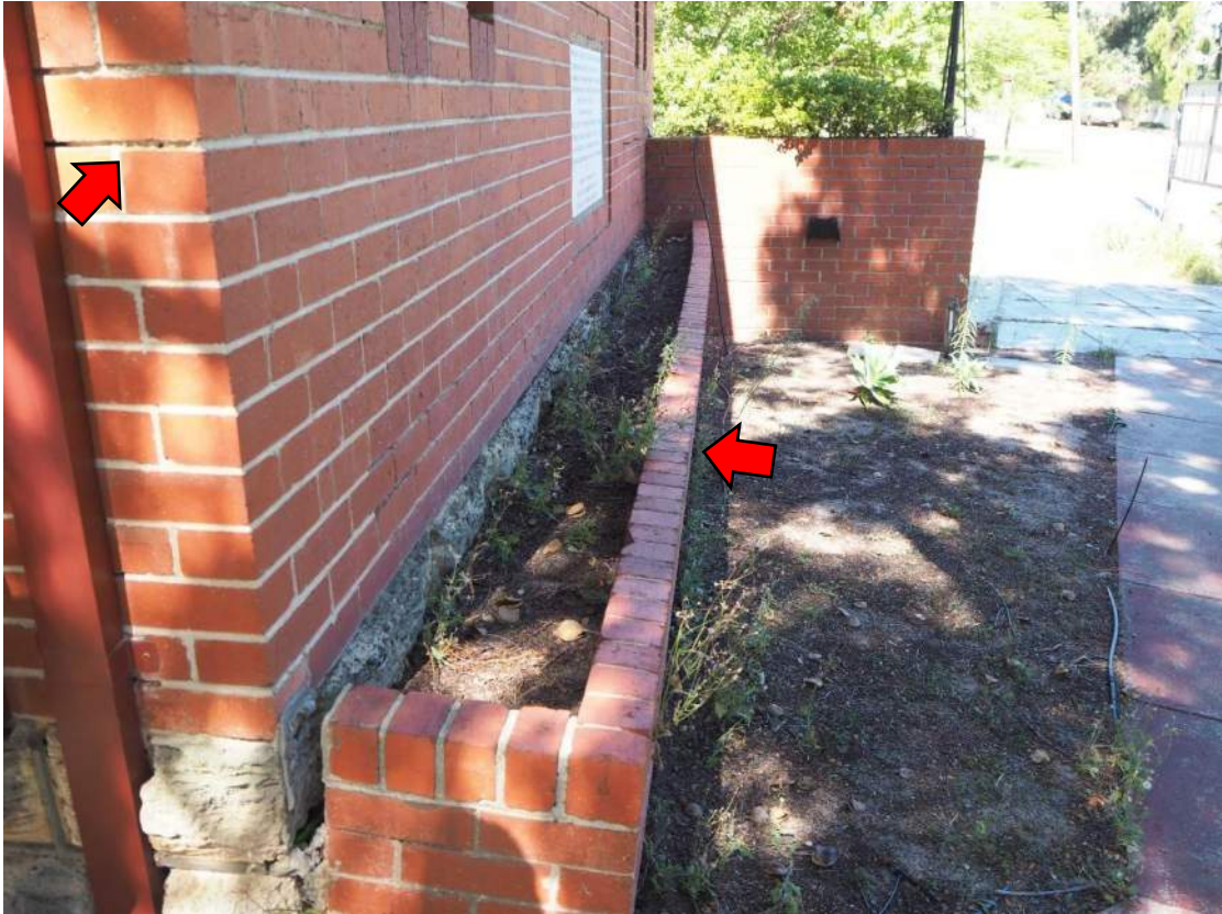
Photo 11 – Planter bed retaining wall has failed. Also note the fretting brickwork
