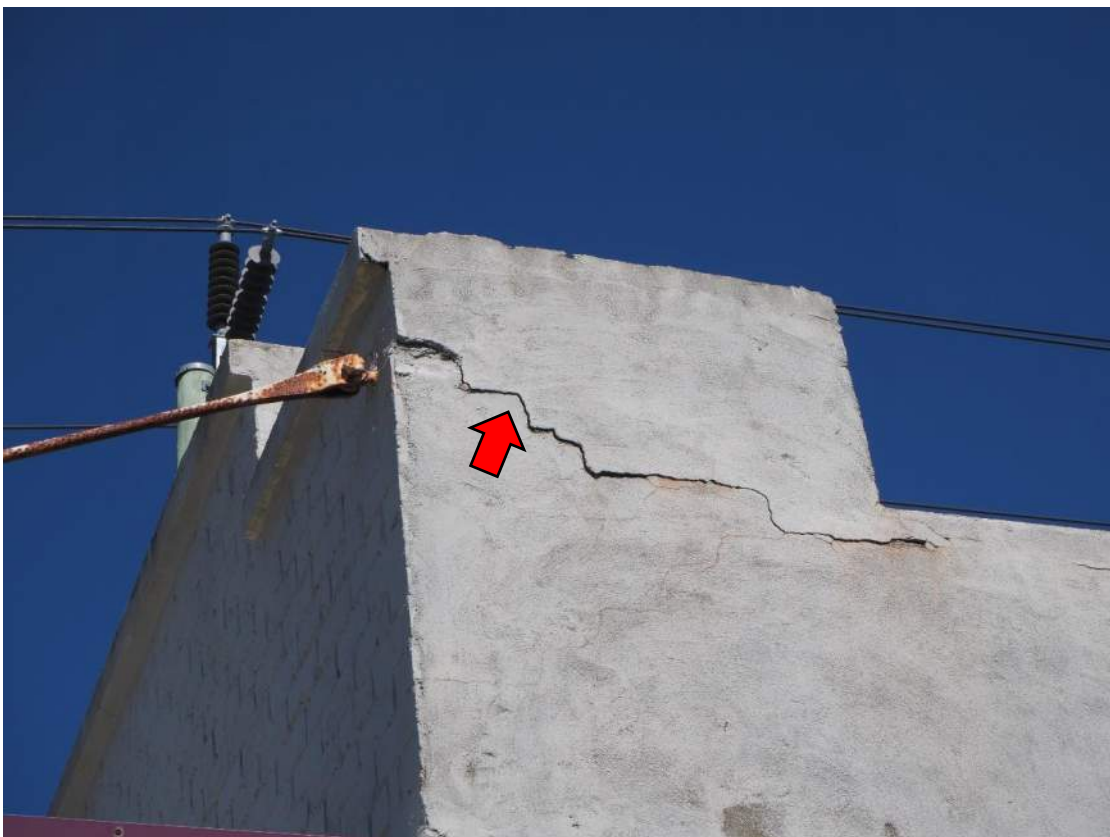
Photo 28 – Crack in parapet caused by awning tie. Awning tie corroding.
