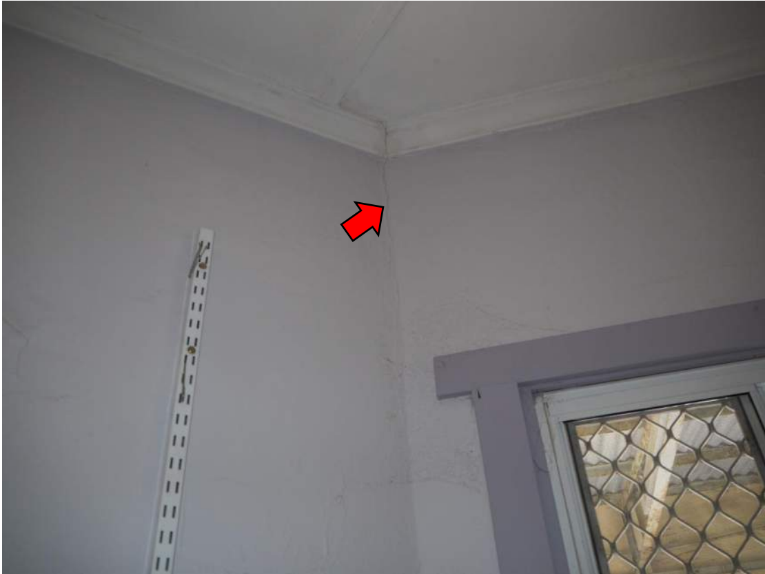
Photo 27 – Minor crack above door to corner shop.
