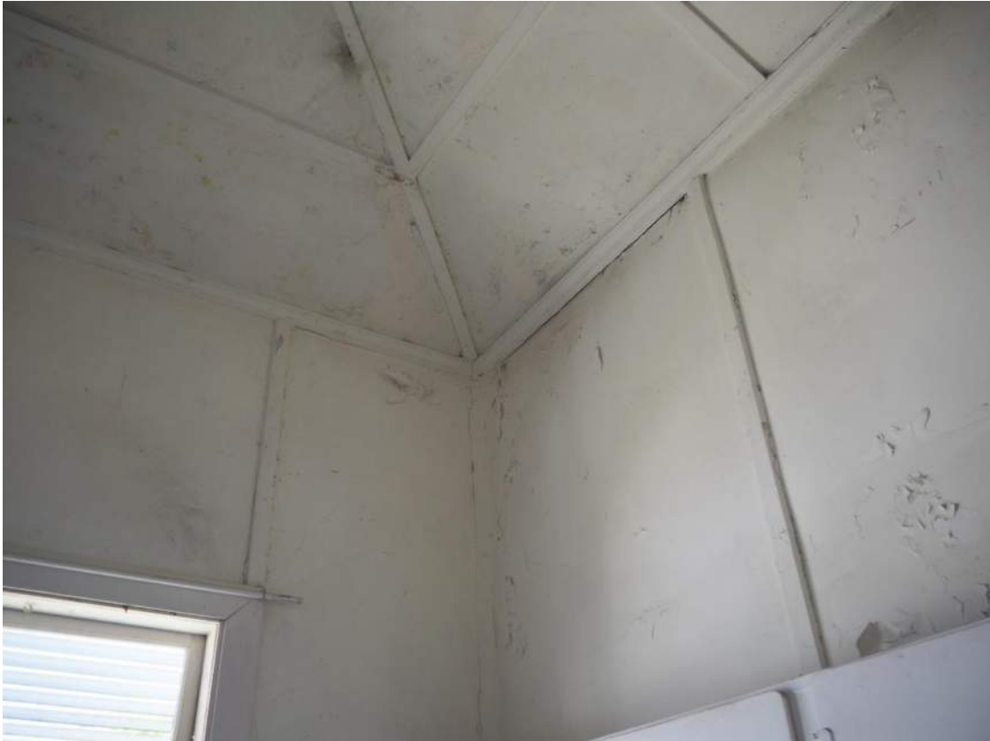
Photo 25 - Internal paintwork on ACM(?) sheets in poor condition.
