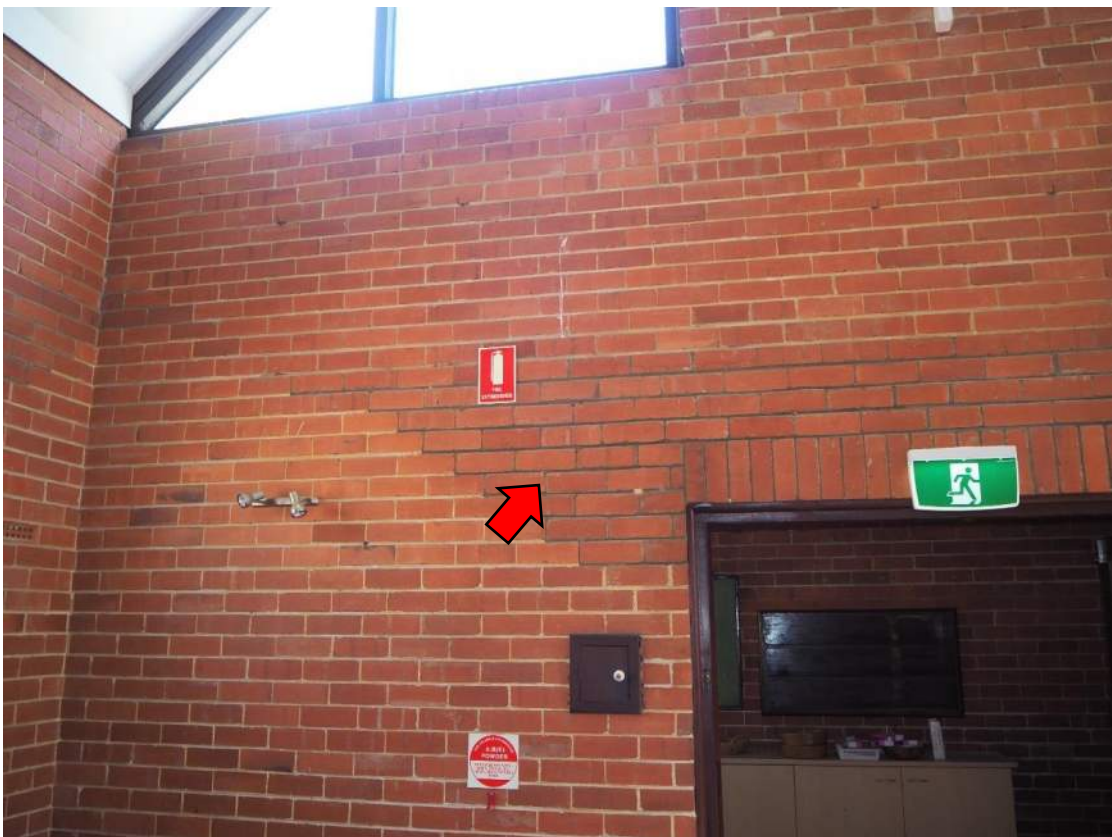
Photo 12 – Different coloured pointing above doorway.
