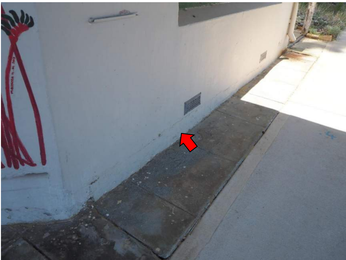
Photo 32 – Cracks and damp damage to base of wall.
