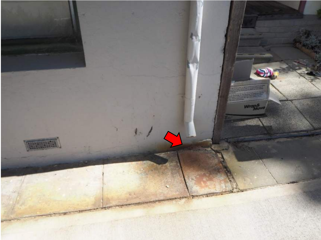
Photo 31 – Downpipe discharging directly onto the ground.
