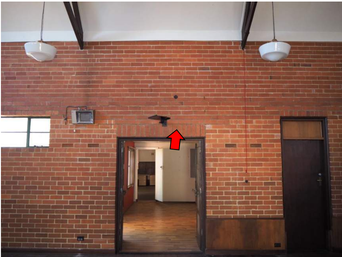
Photo 14 – Different coloured mortar over doorway.
