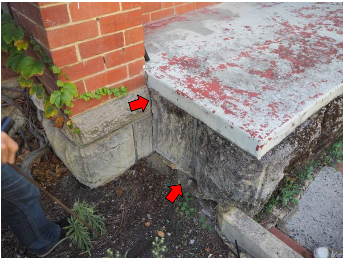
Photo 06 – Step footing blocks undermined and crack opening up between them and the original footing blocks.
