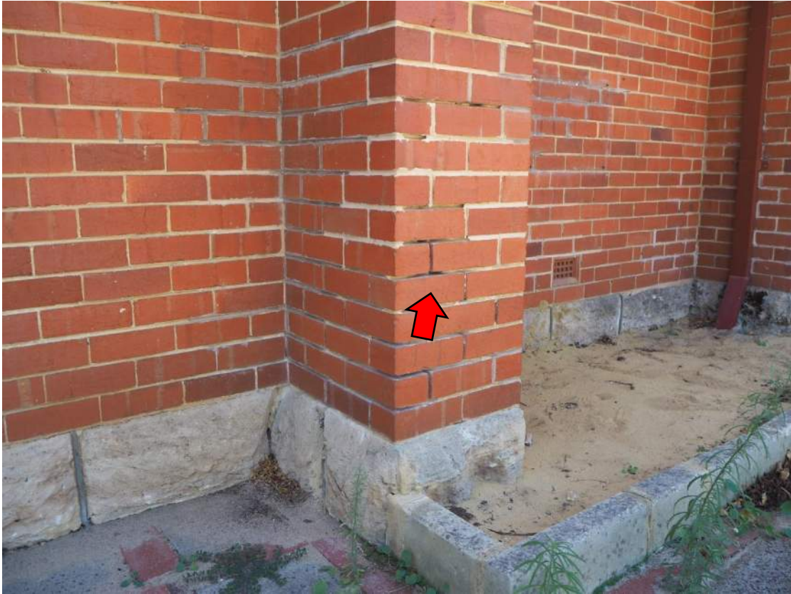
Photo 01 – Fretting mortar, southeast elevation
