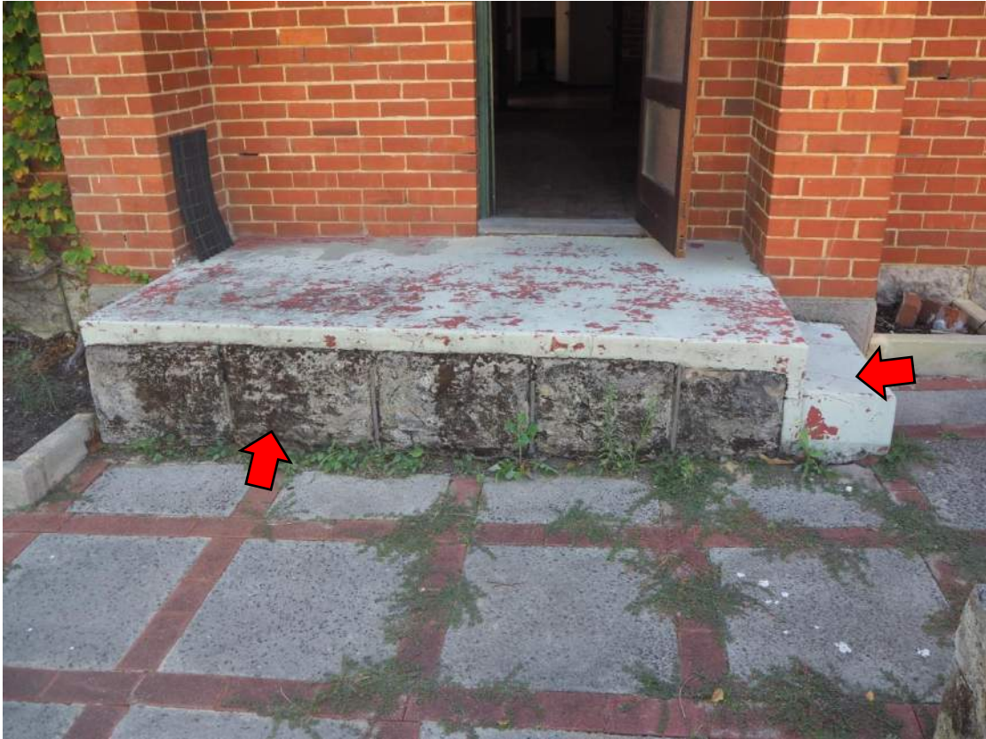
Photo 05 – Entrance steps weathered, and concrete cracked
