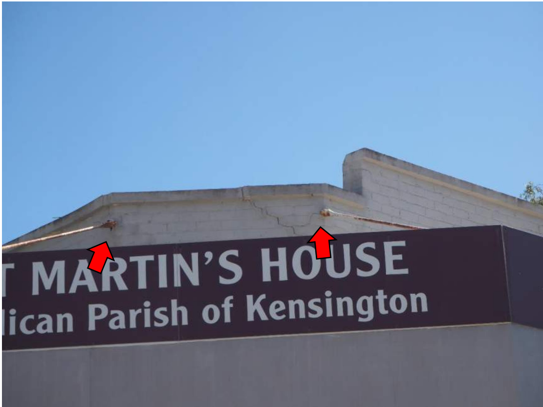
Photo 29 – Cracks in parapet caused by awning ties. Awning ties corroding.
