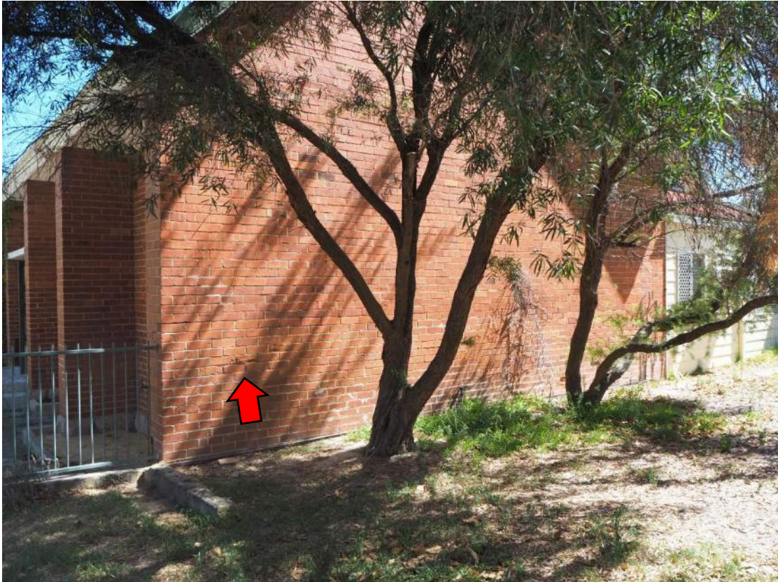
Photo 03 – Fretting mortar, northeast elevation
