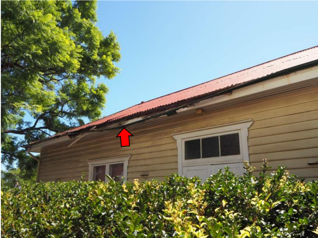
Photo 19 – Corroded and collapsed gutter, southeast elevation.
