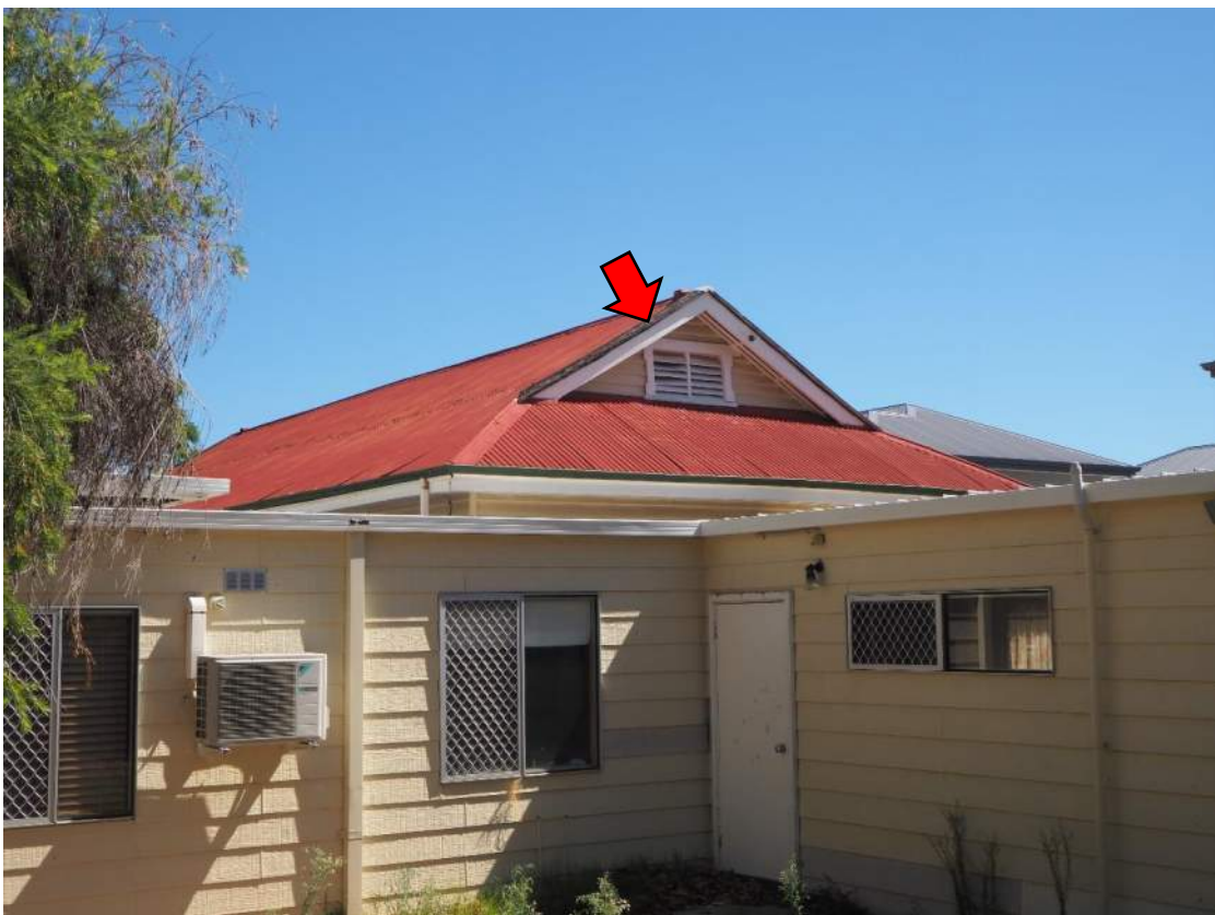
Photo 18 – The roof sheets were in fair condition with some fading. Note the severe weathering of the barge boards on the fascia.
