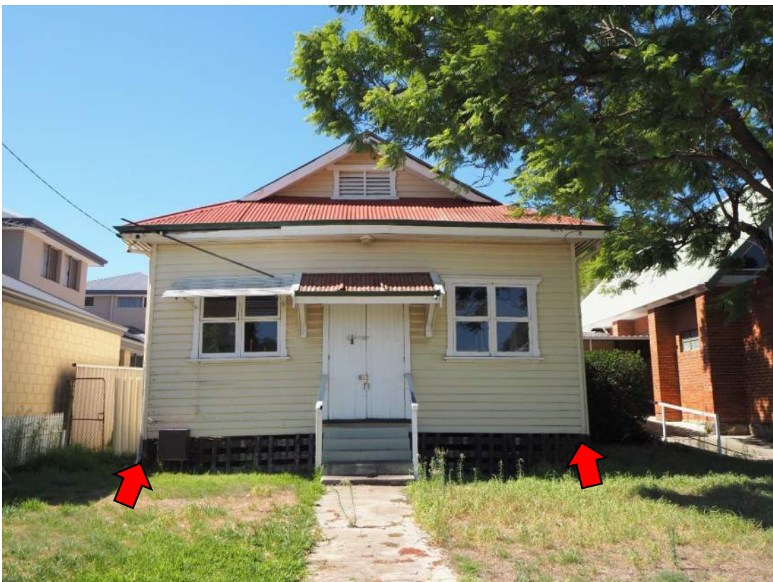
Photo 20 – The sides of the front entrance structure were sagging
