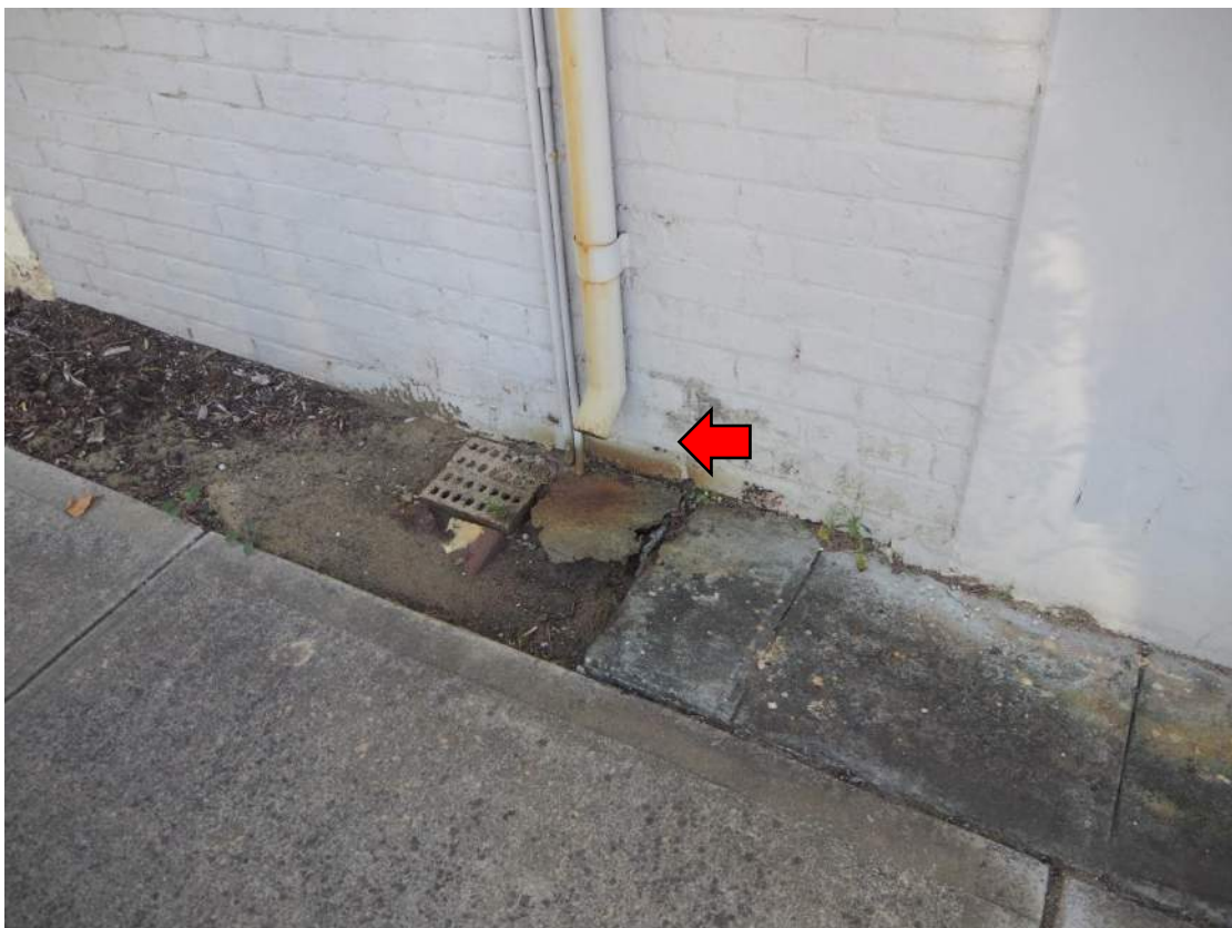
Photo 30 – Downpipe discharging directly onto the ground.
