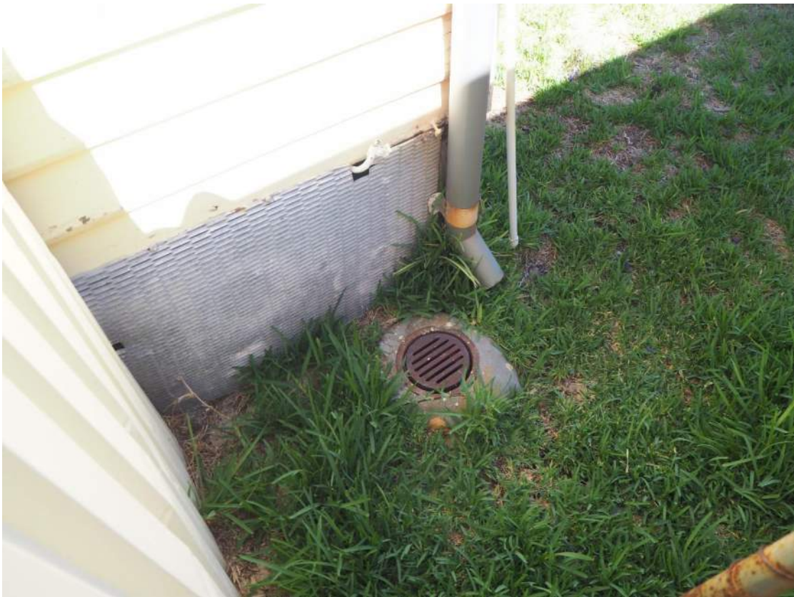
Photo 24 – Downpipe discharging onto the ground
