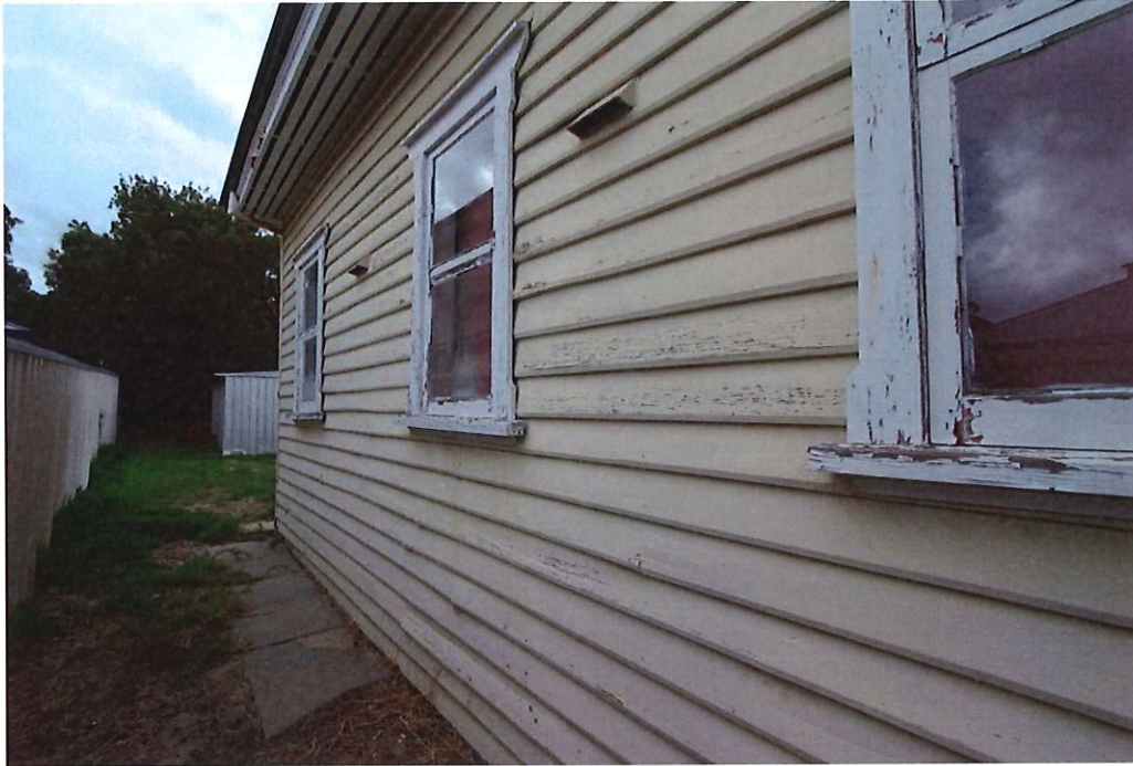
Photograph 13 The western façade of the Hall shows the general level of deterioration of the entire building. Griffiths Architects May 2021
