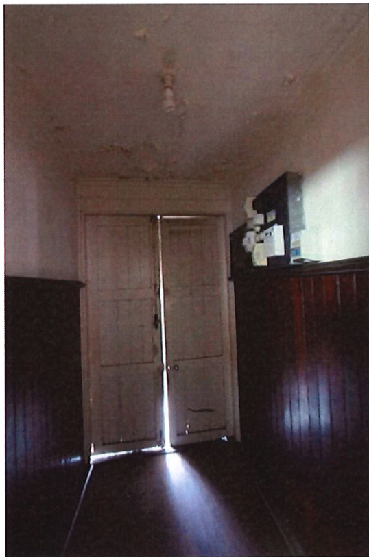
Photograph 14 Interior view of the Hall's wind lobby looking toward the entrance doors. The ceiling shows signs of water damage. Griffiths Architects May 2021
