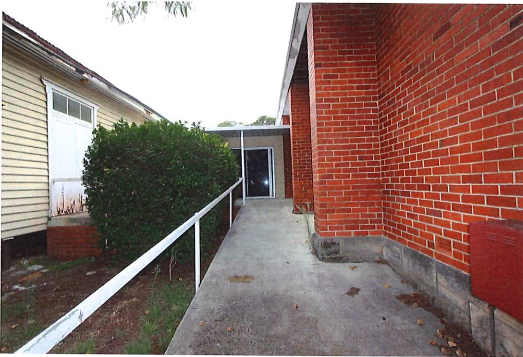
Photograph 7 The ramp between the Church and Hall leading to the entrance of the Link and Hall buildings. Griffiths Architects May 2021
