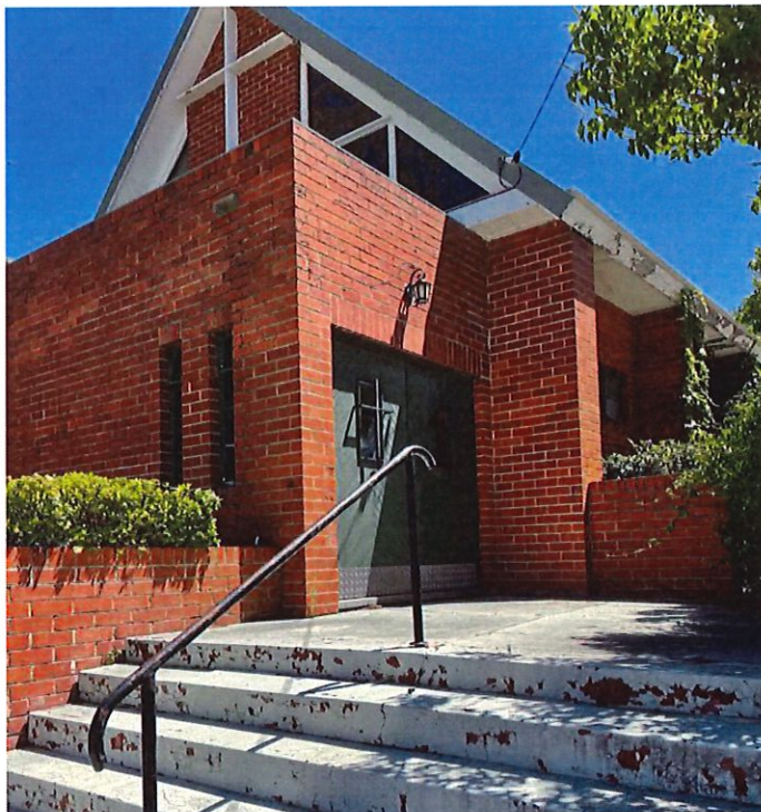
Photograph 2 Painted concrete steps lead up to the double timber with metal cross detail entrance doors at the Church entrance. Griffiths Architects December 2020
