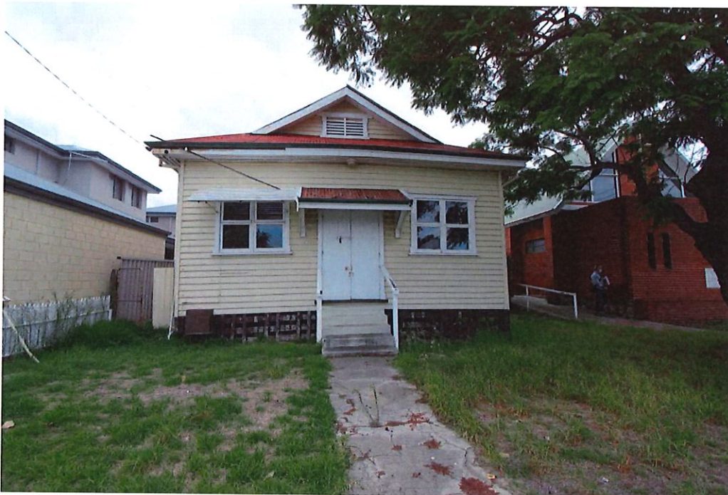
Photograph 12 Dyson Street elevation of Durbridge Hall. The corners of the building are sagging. Griffiths Architects May 2021
