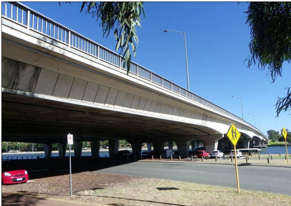
The three Narrows Bridges , with public car parking beneath. (Gina Fraser, City of South Perth, December 2014)
