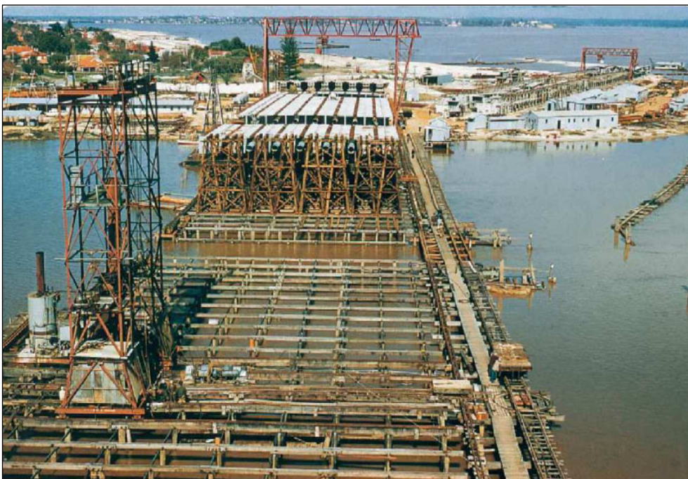
The original Narrows Bridge under construction c1957. (Photograph reproduced with kind permission of Engineers Australia (Western Australia Division))
