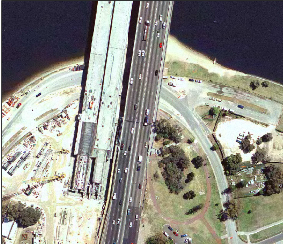
Aerial photograph of the southern (Mill Point) end of the Narrows Bridge showing the duplicate bridge under construction, while the original bridge is still in use. 2000. (City records)
